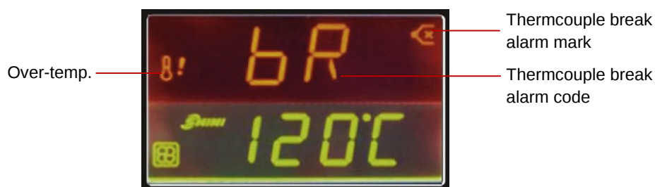
Picture 4-3: Wrong Codes Remark
